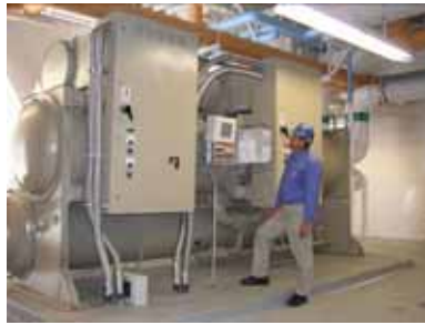
Dual Compressor Centrifugal Chiller
